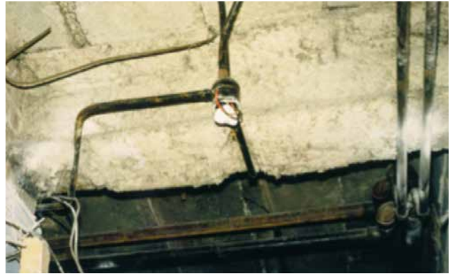
Sprayed coating applied to structural steel. Note damage around the electrical junction box.
