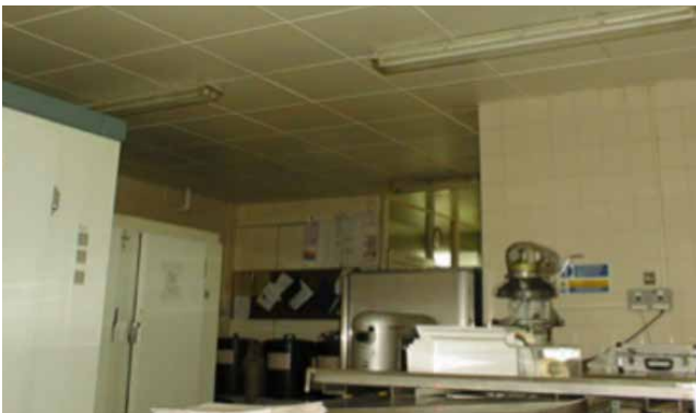
AIB as a firebreak in a ceiling void.
