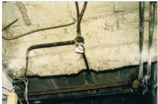
Sprayed coating applied to structural steel. Note the damage around the electrical junction box.
